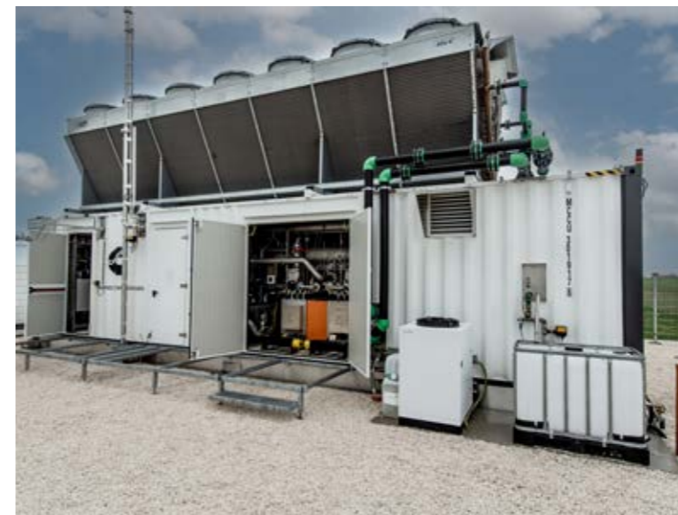
2 MW water electrolysis in Rubensdorf
